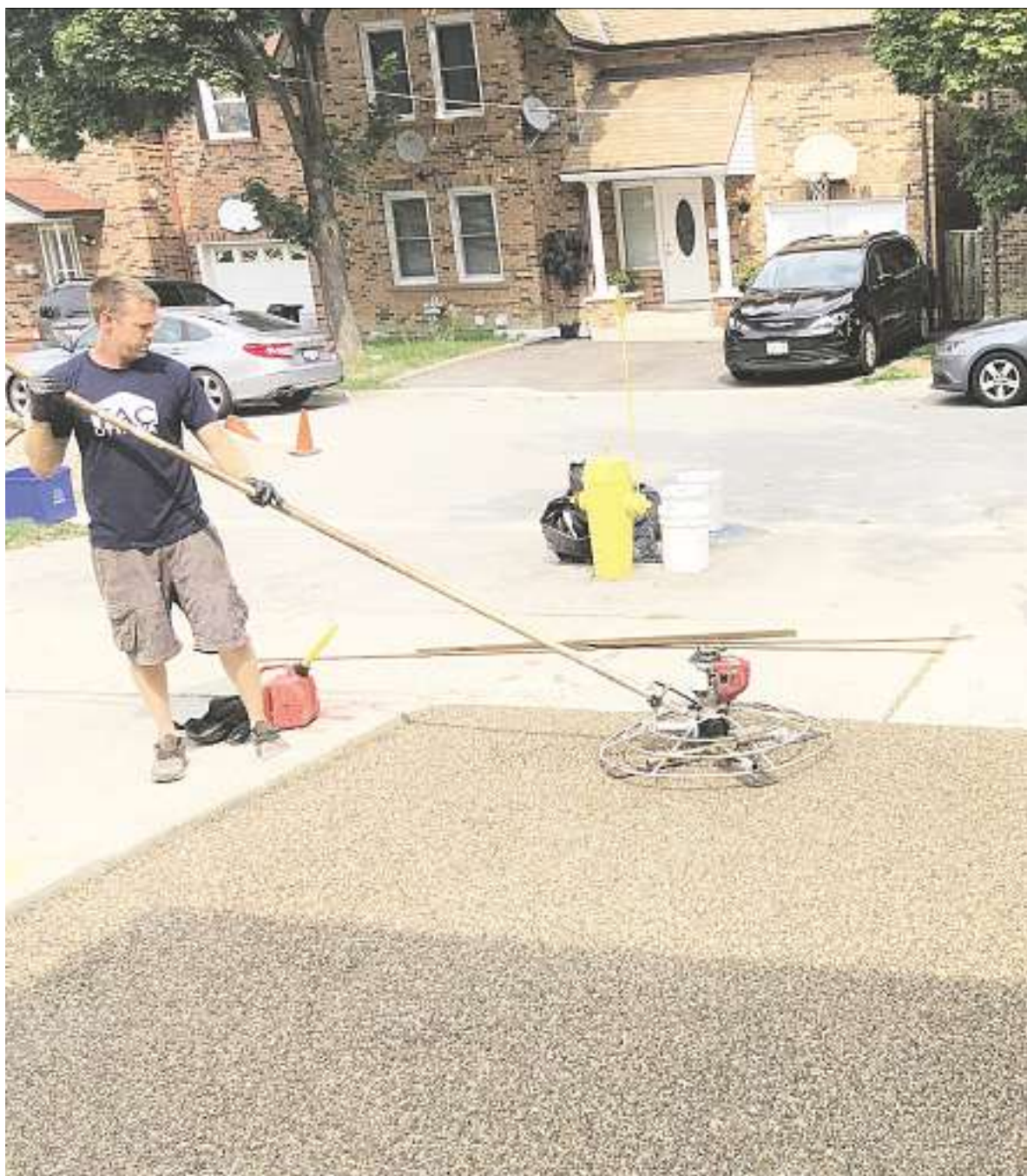
Etobicoke homeowners saw how concrete driveways had heaved and broken apart due to spring thaw and were drawn to the elasticity of the PurePave surface. PHOTOS: PUREPAVE
