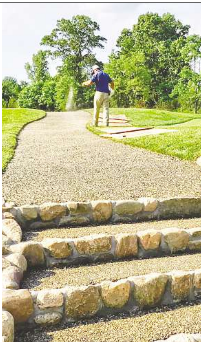
This golf cart pathway for Manhattan Woods Golf Course was built with gravel to eliminate costly water damage.
