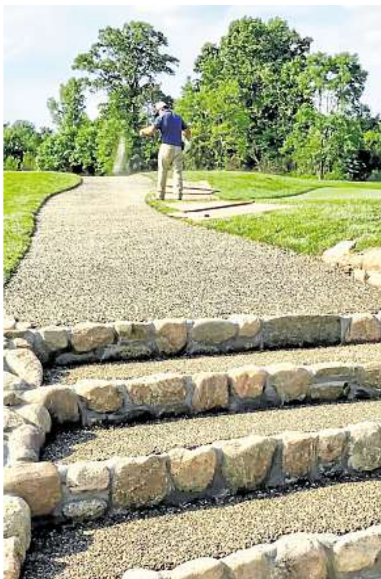
This golf cart pathway for Manhattan Woods Golf Course was built with a goal to eliminate costly water damage.
